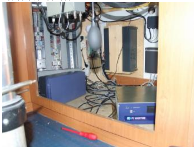
Figure 5 Boxes and wiring
